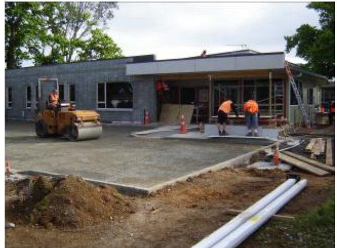
Blockwork to the front of the Dental Clinic is complete and the car park is ready to be poured.
