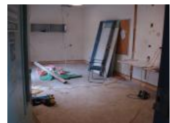
The removal of a wall has resulted in a larger Nurses Station.
