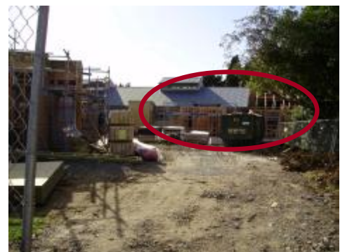
The foundations have been laid and framing commenced for the Intensive Care Area (ICA)
