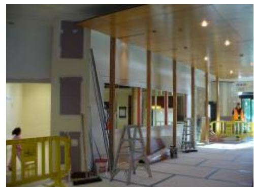
A new patient waiting area will be on the other side of the wall (shown above).
