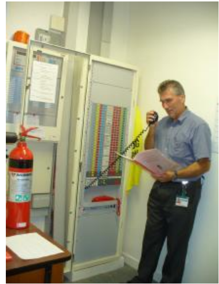
Terry carries out safety checks from the Fire Room
