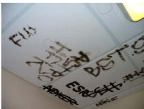
Graffiti on the ceiling of a Kidz First public toilet
