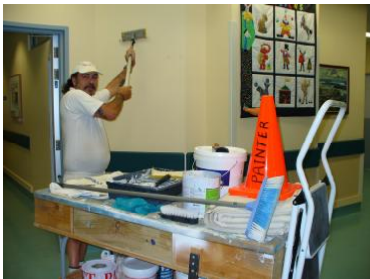
“Good as new” – Norm the painter cleans up some of the Graffiti in Kidz First
