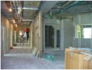
The box marks the Reception area. The photo also shows a Ward corridor.
