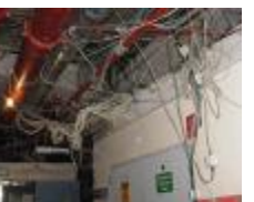
Amazing amount of wiring and cables
