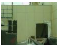
The plant room is being built above the Cardiac Cath Lab. Equipment will be lifted in by crane.
