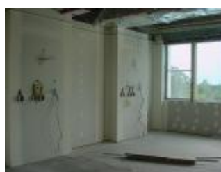
Service panels in a Level 2, 4 cot bay
