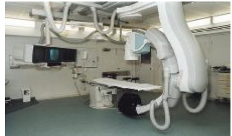
An example of the catheter laboratory equipment. A decision will soon be made by CMDHB on the brand of equipment it will purchase
