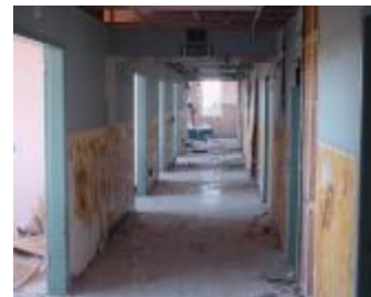
March 22nd - walls still intact
